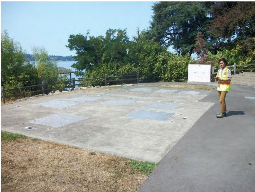
Pump Station 4 with access from Lake WA or land
